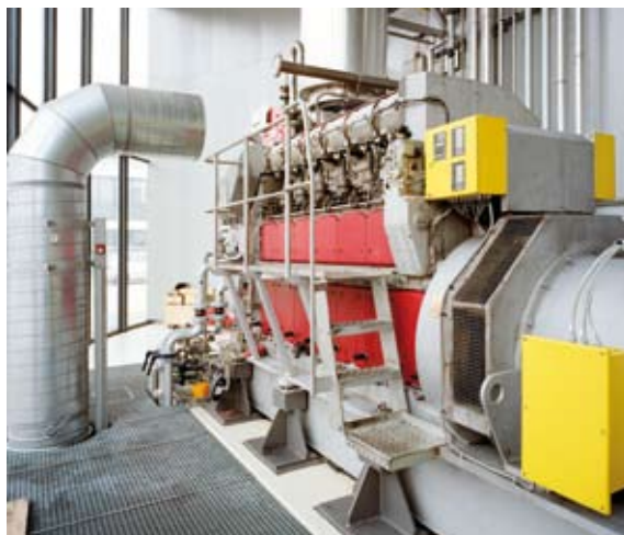
The 21/31 bio-fuel engine and generator
