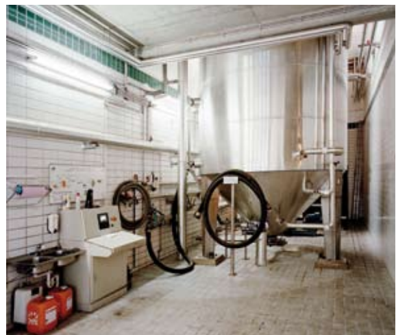
Fuel conditioning separator
