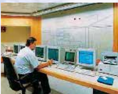
7 Pipeline Station Control Room
