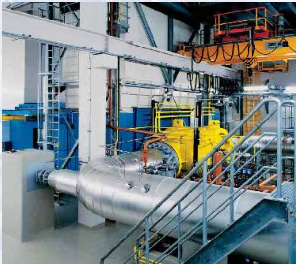
9 Inside the Werne Facility
