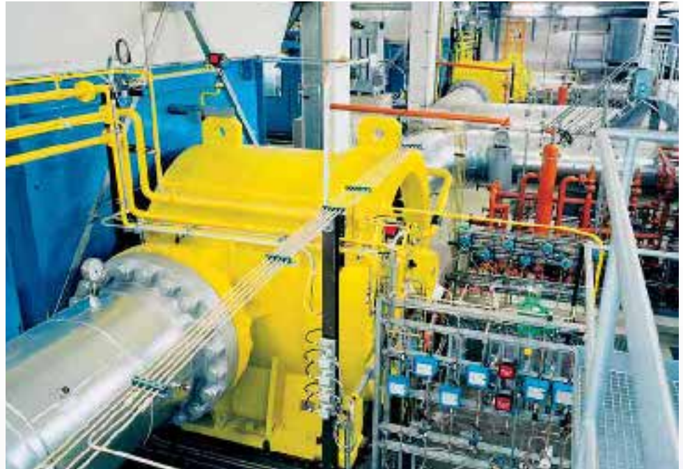
6 RV090 Pipeline Compressor
