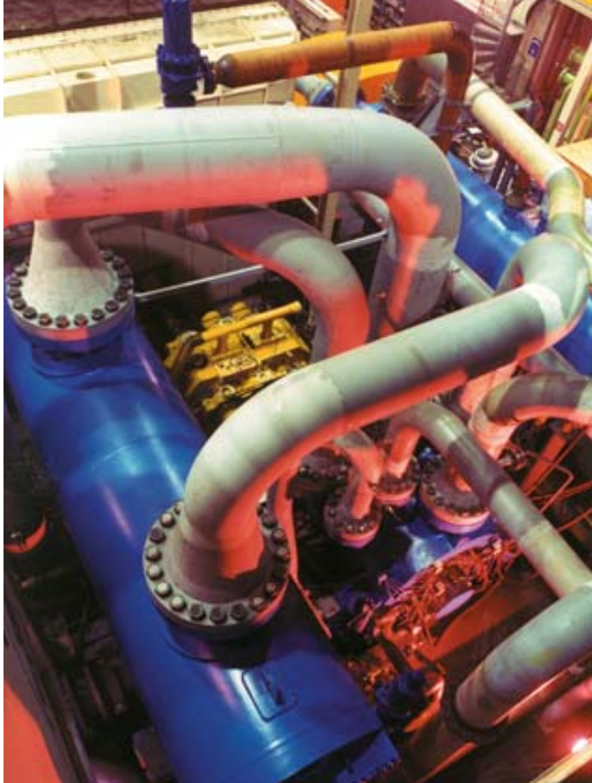
Fig. 16: Arrangement of HP Compressor for Full Load Test
