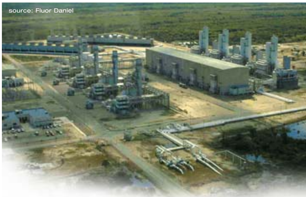
Fig. 3: Nitrogen Production Plant
