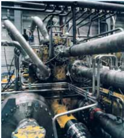
5 Compressor in the field during Class I test
