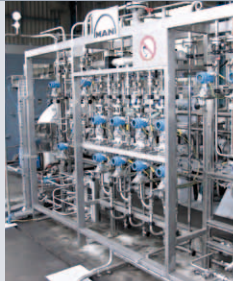
New dry gas seal instrumentation and monitoring rack
