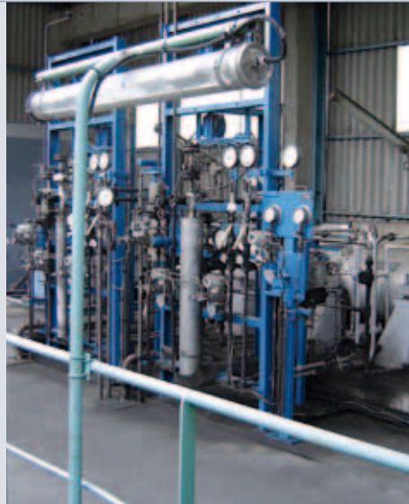
Old oil-lubricated shaft sealing instrumentation and monitoring rack
