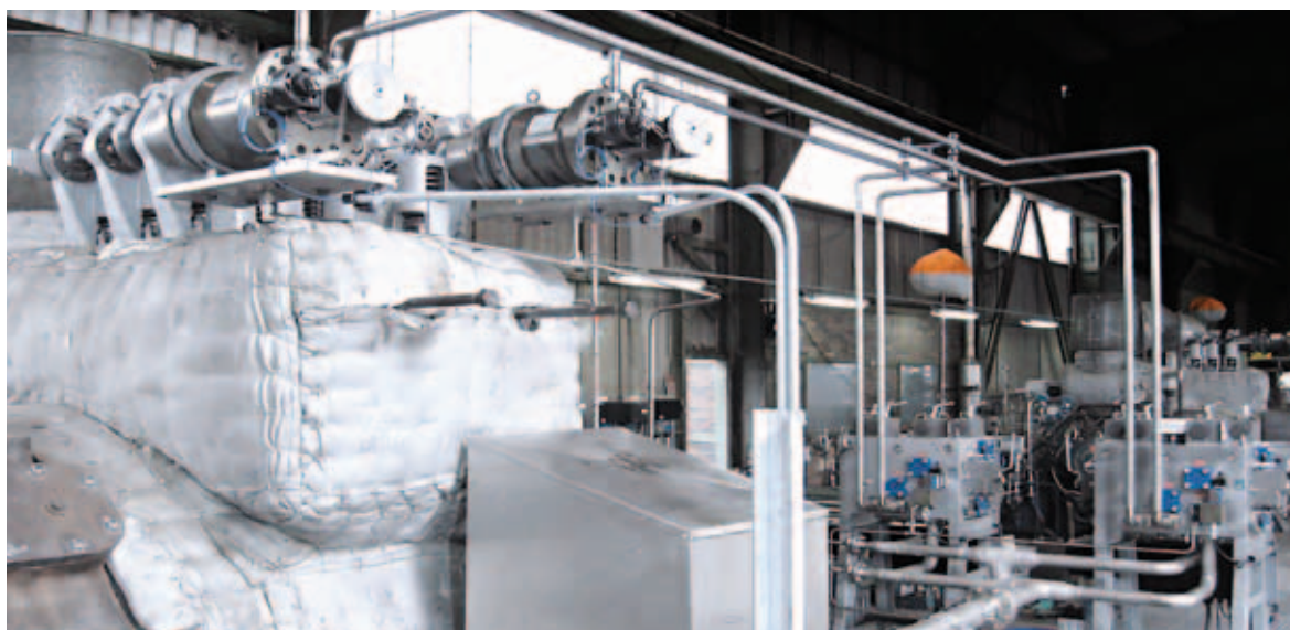
Steam turbine type DEK 710 equipped with the newly designed speed control system
