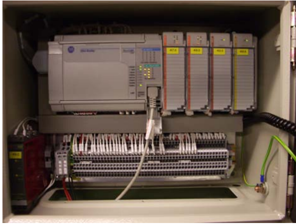
New control box
